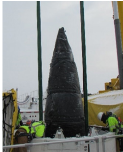
Initial lift of GBI from silo for MDA's Service Life Extension Program (SLEP).
